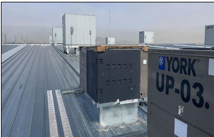
HVAC systems are installed on the roof.
